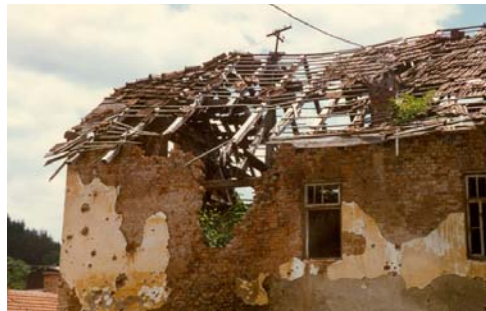
Destroyed Bosnian House (Photo: J. Riggs)
